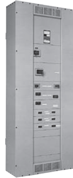
Circuit Breaker Distribution Panel Type P4/P5
